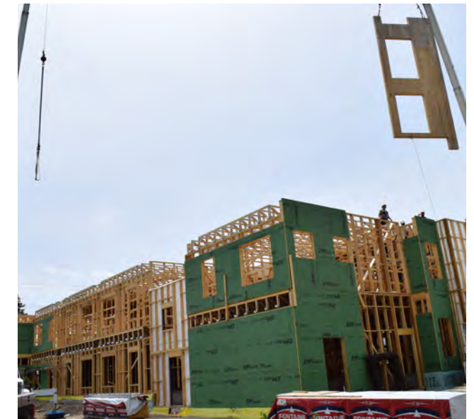
Cross-laminated timber, a value-added and climate-friendly construction material in lieu of steel, is used during construction of a 40-unit apartment building in Portland in summer 2020.
