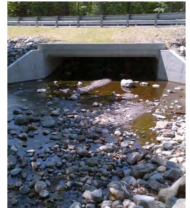
This stream crossing on Bottle Brook in Kingsbury Plantation is an example of a climate-ready infrastructure project that is also geared to improve habitat connectivity.
